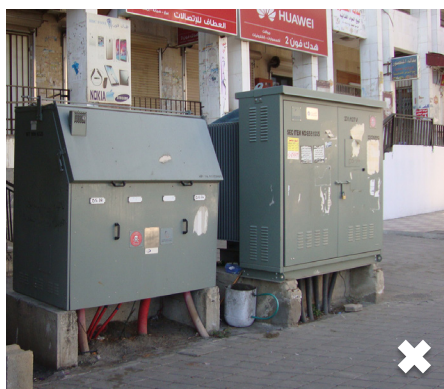
Figure 175 Exposed utilities on sidewalk
